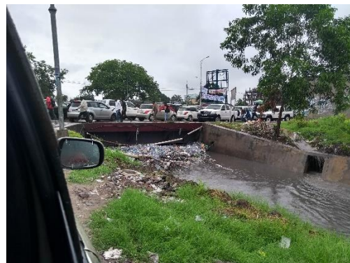
Figure 5: Flooding in Kinshasa, attributable mainly to blocked drainage channels and rivers, killed 45 people in a week in January 2018 and was followed by a deadly outbreak of cholera
